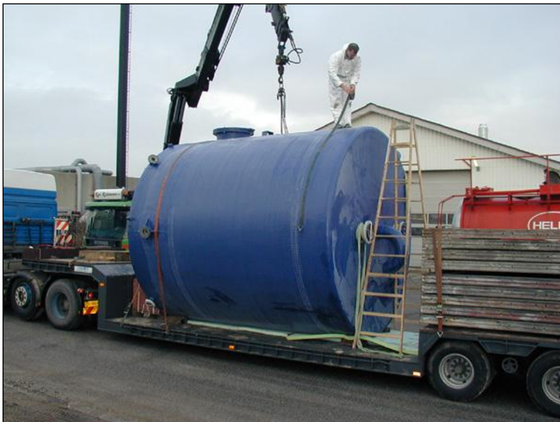
Customer: Energi E2, Denmark
